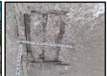
Large Spall in Soffit – Exposing Rebar
